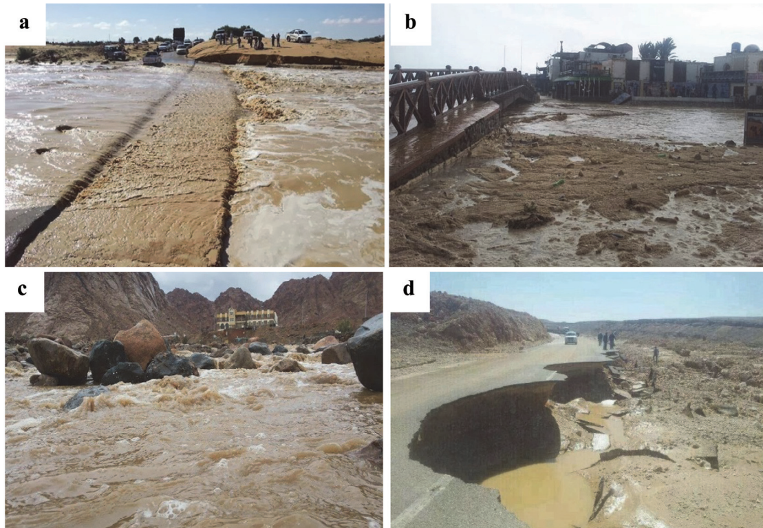
Fig. 9. Damages of the 9/3/2014 flash floods: a. Central Sinai, b. Saint Catherina, Southern Sinai, c. Daniela Village, Dahab, and d. Hurghada highway collapse.
